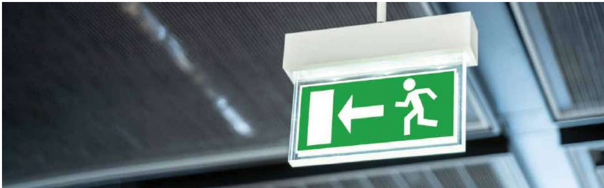
Centralized Monitoring EXIT Sign
