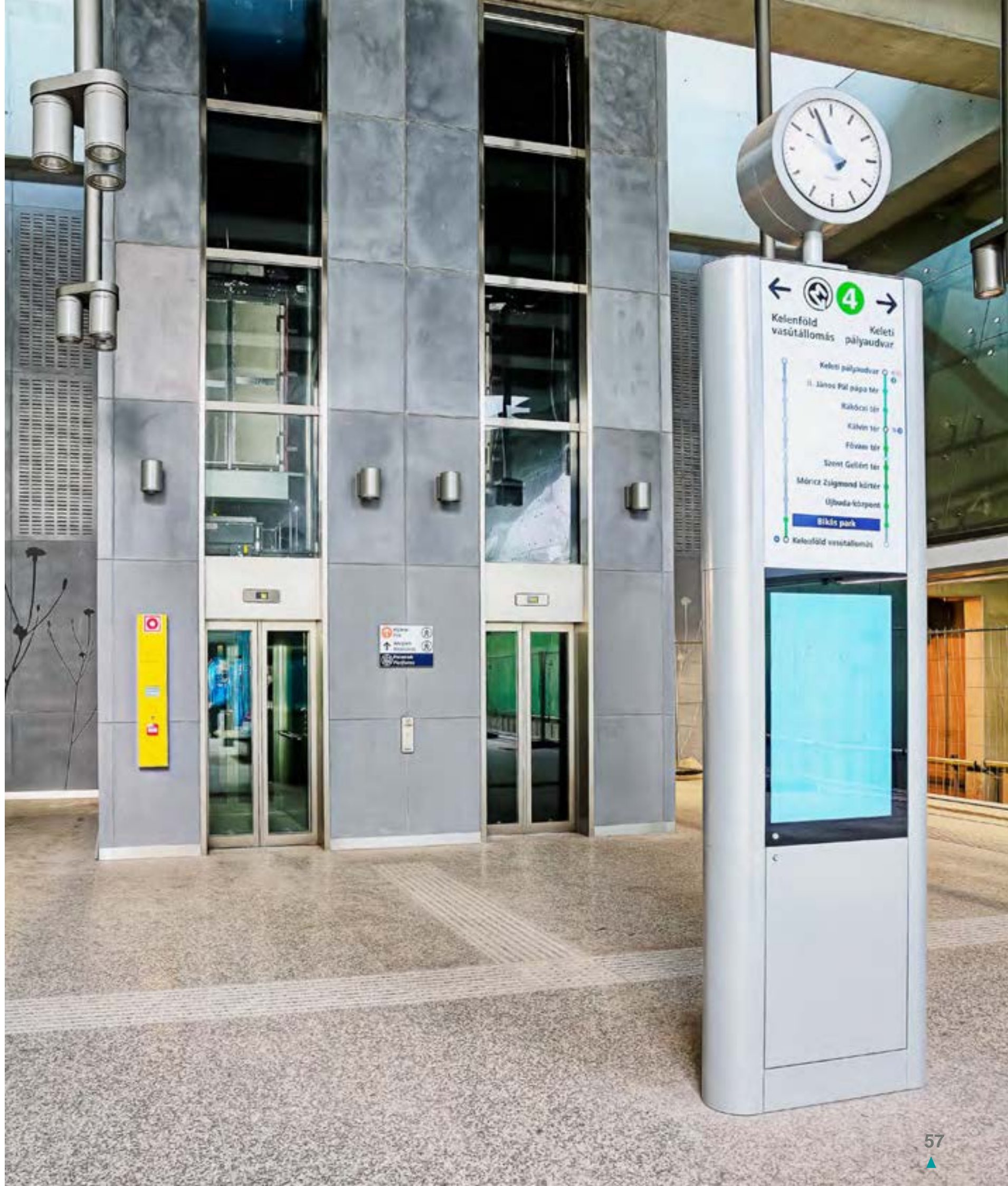
ELEVATORS INSTALLED AT BIKÁS PARK STATION
